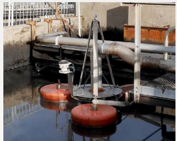
An Ultra-SurfCleaner operating in an API separator.
