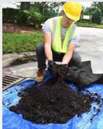
Actual contents of a 2-month Drain Guard test.
